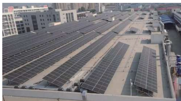
Tianjin base PV power project
