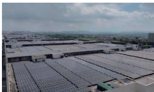
Qingyuan base PV power project
