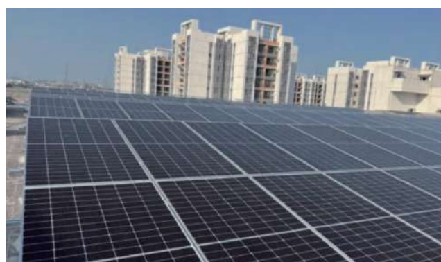
Guangzhou Headquarters PV power project
